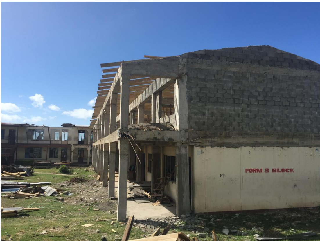
Photo – Cyclone damaged high school, Ba Fiji (taken by Prof David Smart, May 2016)
